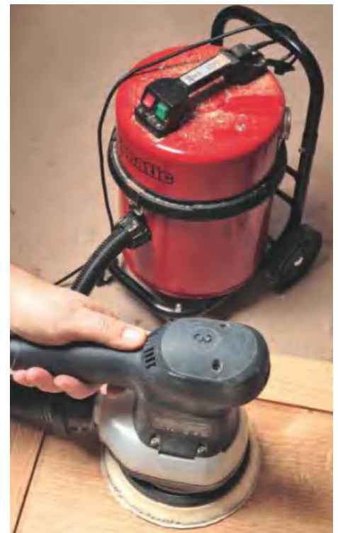
▲ Pic.13 Sanding dust needs to be collected at source otherwise it gets everywhere
